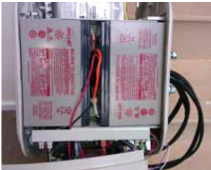
BATTERIES ROTATED BACK IN PLACE
